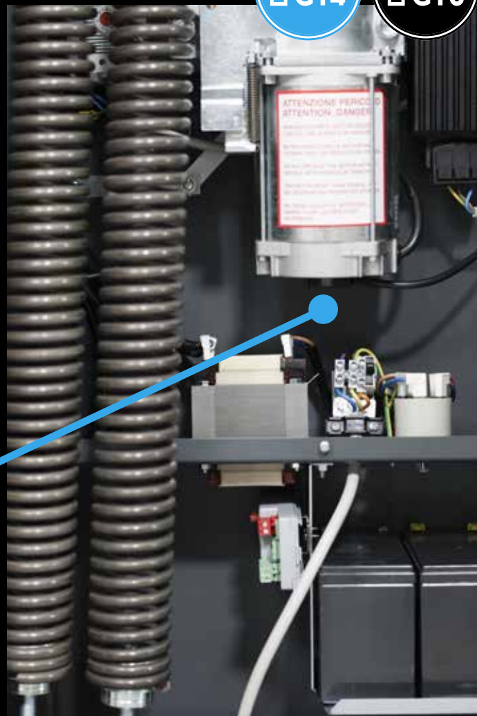
Encoder pictured at the base of the motor.
